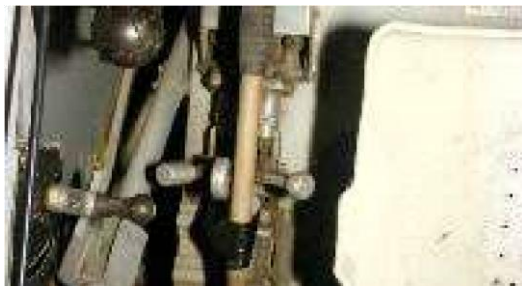
Cockpit Hydraulic Controls Victoria
